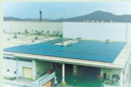
Solar panels at the Shiga Plant
