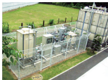
Decentralized water treatment & supply system
