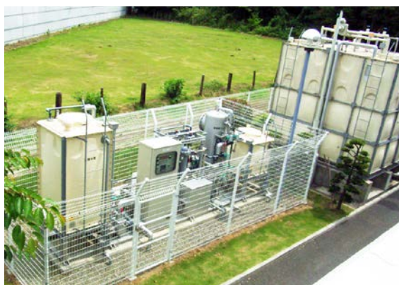
Decentralized water treatment & supply system
