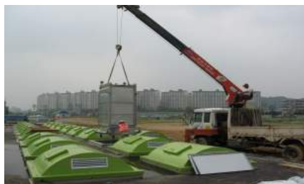
Large scale water treatment facilities in Korea
