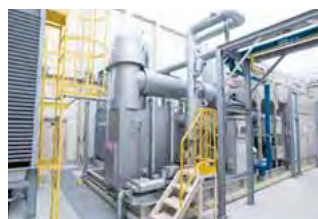
Nagahama Plant's co-generation facility
