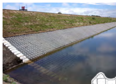
Kawauchisawa River with GOBIMAT installed
