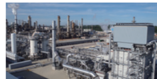
HyCO* plant for hydrogen supply
