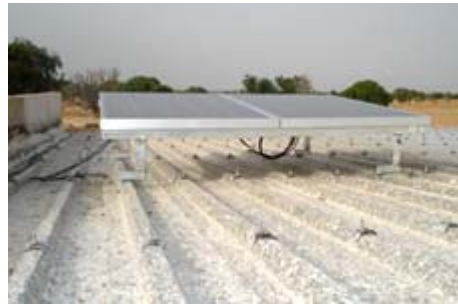
Solar panels installed on the school's roof Photos: Plan Japan
