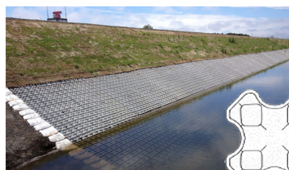
Kawauchisawa River with GOBIMAT installed
