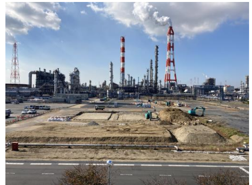
Construction of a chemical recycling facility at the Ibaraki Plant is in progress.
