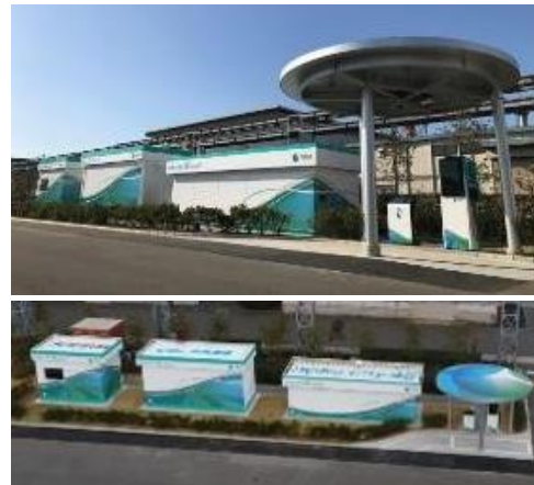
Hydrogen station in Kawasaki
