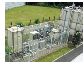
Membrane filtration system for groundwater
