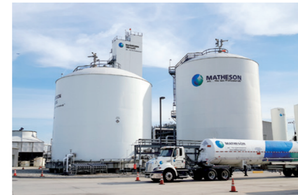
Industrial gases, industrial gas-related equipment and facilities
