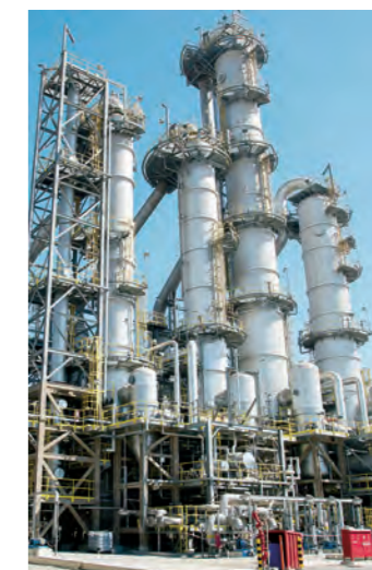
MMA monomer plant with the world's top-class production capacity that has started operation (Saudi Arabia)
