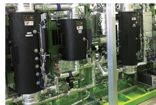
Small-scale pilot plant for the production of light olefins
