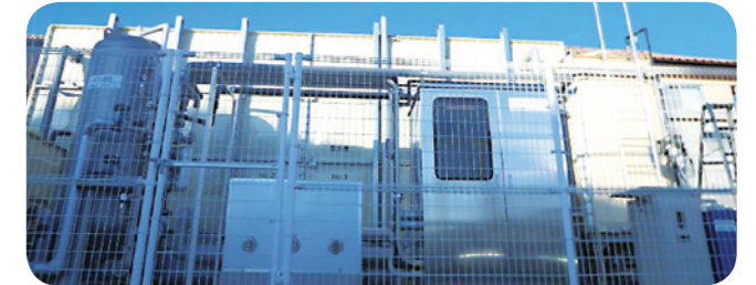
Groundwater membrane filtration system that continued to operate during the Kumamoto Earthquake (Musashigaoka Hospital)
