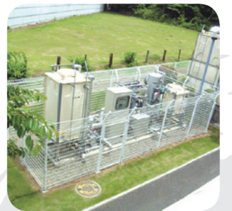
Groundwater membrane filtration system
