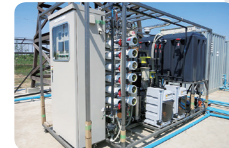
RO unit for desalination
